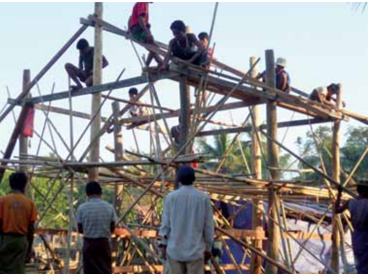
▲ Trainees building a disaster resilient home as a demonstration during their carpenter training organized jointly by UNDP and UNHABITAT in Thailand. (UNDP)
